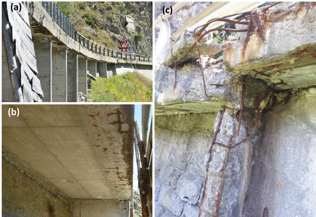
Figure 6. Presentation of Bridge III and observed damage. (a) Presentation of the bridge; (b) Damage on the slab and kerb; (c) Damage on Pier I.
